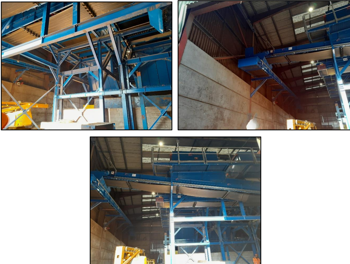
New processing plant installed within building (non-operational)
